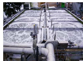
The PRO 2 AIR Pre-PUR ® membrane tube diffuser from NORRES in operation
